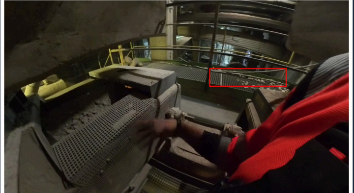
Inspect Belt Condition on Gypsum Scale 535-DB2
