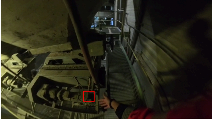
Verify Motor Cooling Fan on Belt 535-DB3
