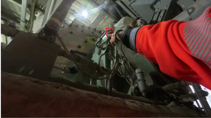
Verify Oil Flow Meter Indicator Position
