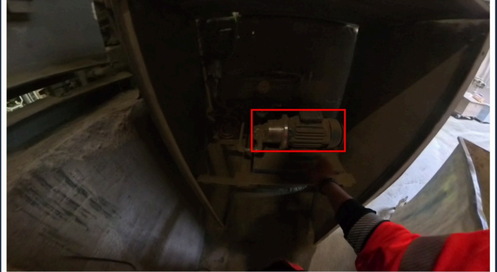
Inspect Lube Pump 565-SM1 and Pressure Gauge
