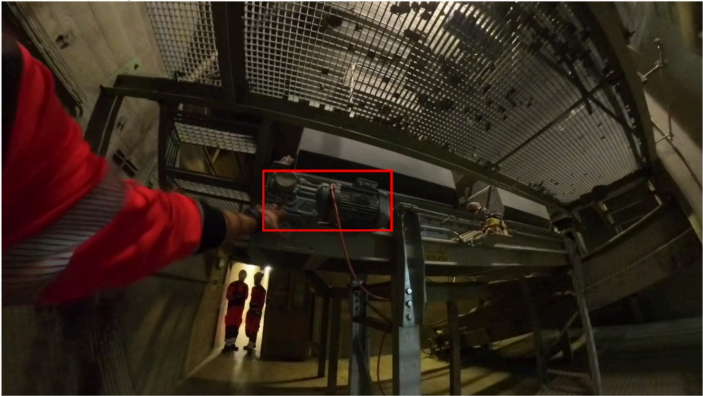
Inspect Geared Motor on Belt 535-DB5
