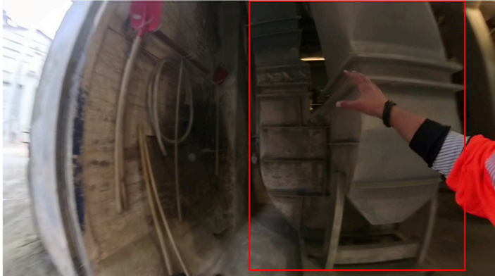
Inspect Fan 565-VE2 Casing for Dust Leaks
